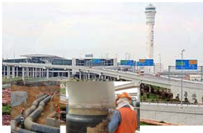
Chilled Water Piping from Chilled Water Plant to Development in KLIA 2 Including KLIA 2 Terminal, Sepang, Selangor
