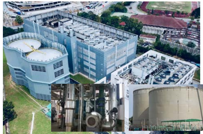
GDC Chilled Water Thermal Energy Storage Plant, Putrajaya (ACEM Engineering Award 2015 – Bronze Award of Commendation)
